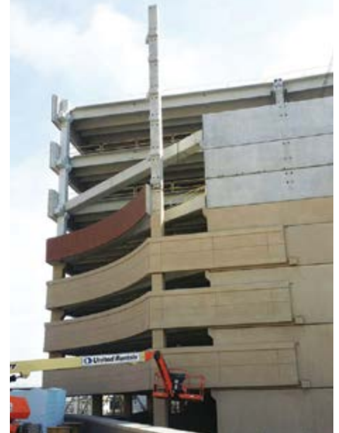
The design-assist format aided the fast erection, which took less than 4 months to complete in early 2016.
